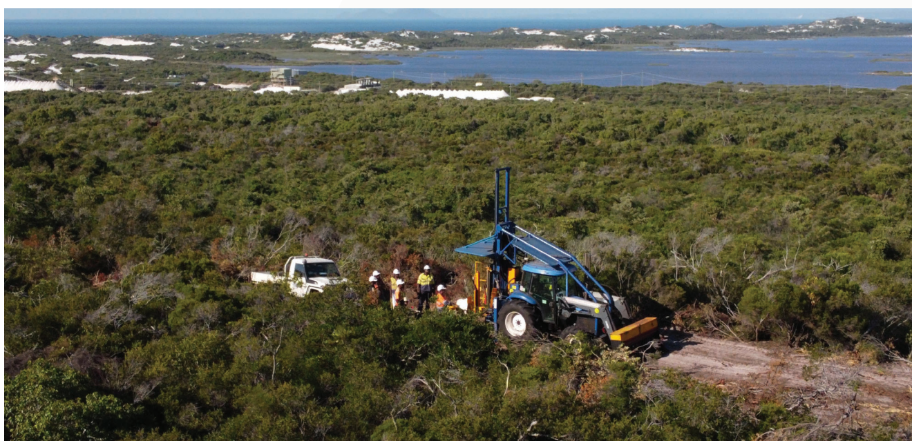
Figure 4: CFS project August 2021 drilling with vacuum drill rig (Mitsubishi operation in the background)
